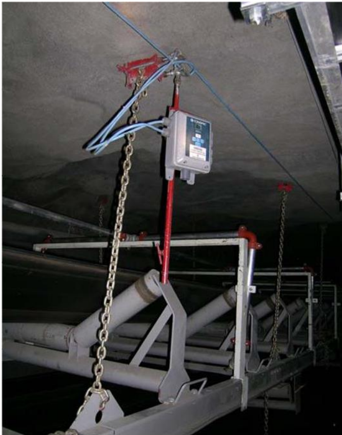
Figure 2 - Properly installed CO sensor
